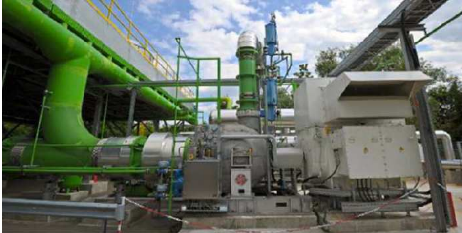
Fig.5. 2,3 MW generator using HDR technology in Landau, Germany.
